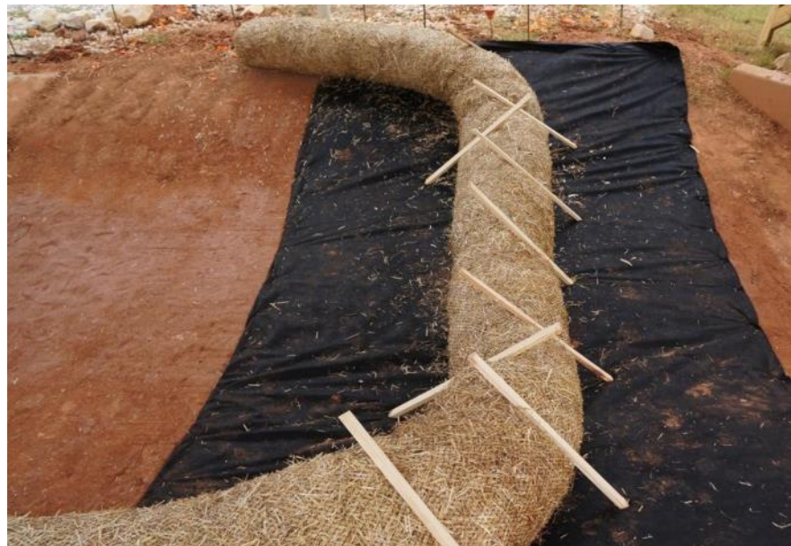
Figure CD-4 Wattle Check Dam (ditch check) (Photo courtesy of Auburn University Erosion and Sediment Control Test Facility)
