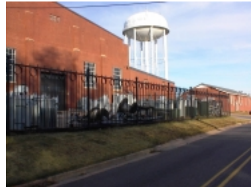
An Orderly, Clean Transformer Yard at a Municipal Facility
