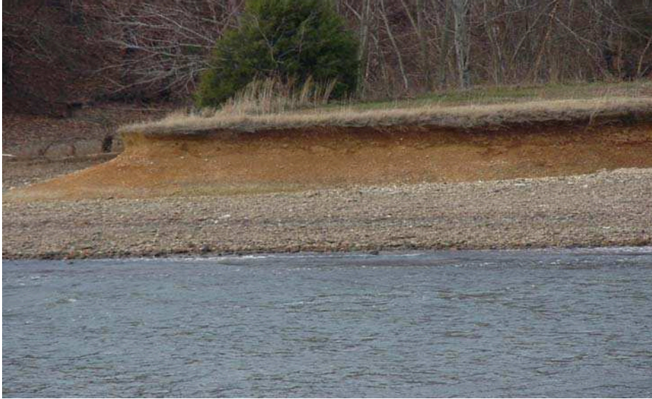
Left: Eroded shoreline prior to stabilization.
