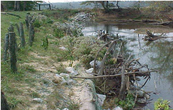
Left: Early stages of willow-stake planting and root wad installation to restore an eroding shoreline on Choccolocco Creek (Talladega County).
