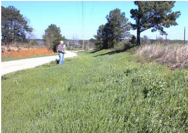
Left and Below Left: Ed Holley, Barbour County District Conservationist, observes McSwain Creek dirt road stabilization sites. Roadside swales have been installed and vegetation is established along this highly erodible dirt road near stream crossings.
