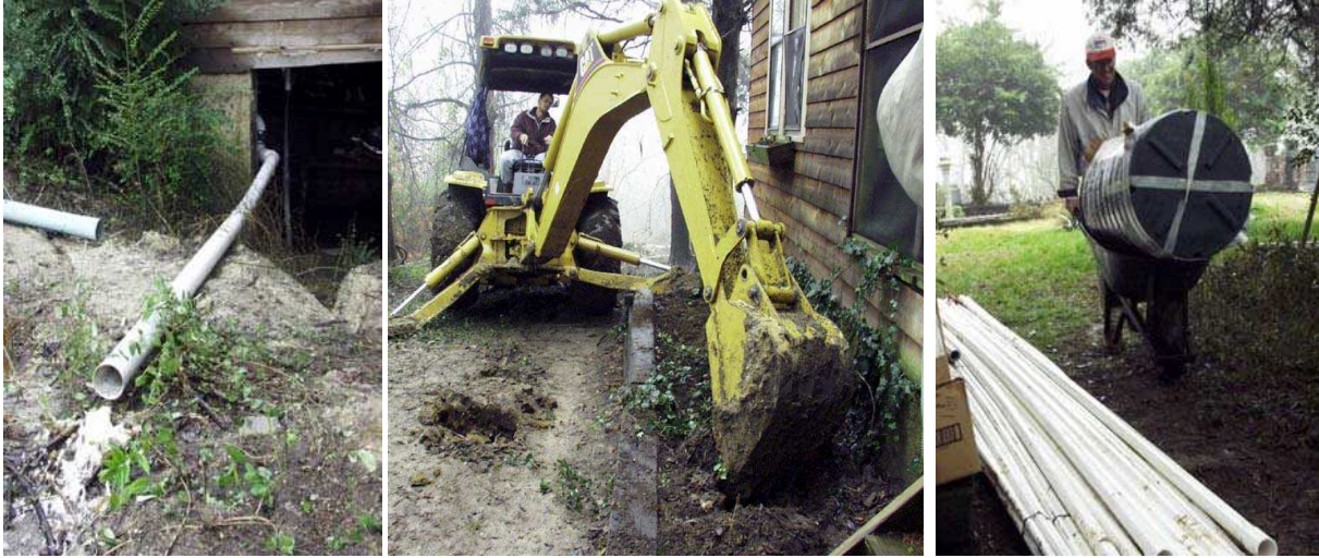
Installation of an alternative onsite wastewater treatment system (drip irrigation tubing) at a Black Belt residence in Sumterville (Sumter County). Note the direct discharge from the pipe onto the ground in the upper left picture.
