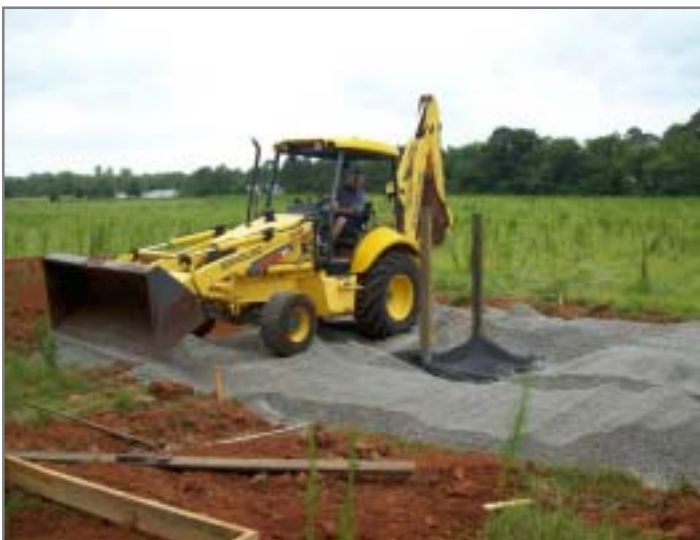
Installation of a watering trough with a pad for cattle in the Harris Creek Watershed
