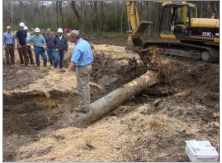
Darrell Westmoreland, North State Environmental, Inc., describes placement of a log vane structure in the newly constructed stream channel.
